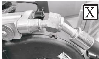
Improperly Seated O-ring Land
